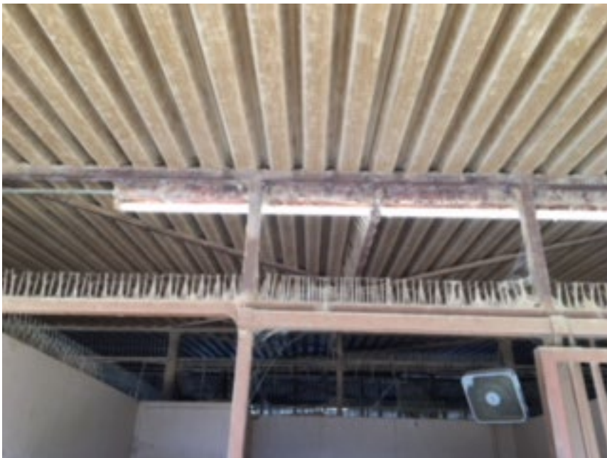
Light fixtures with cobwebs collecting dust.
