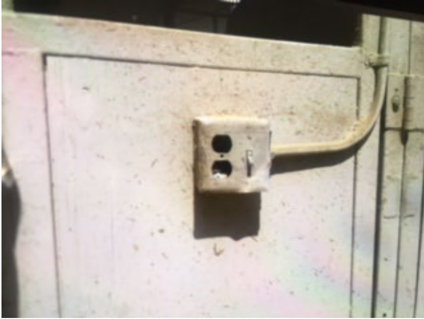
Fix, replace or remove exposed electrical outlet
