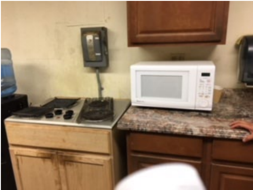
Utility may need to be removed, presently located directly over the range / cooker
