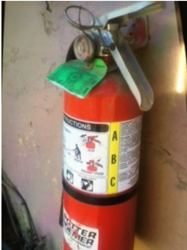
Green tag is torn in half.
