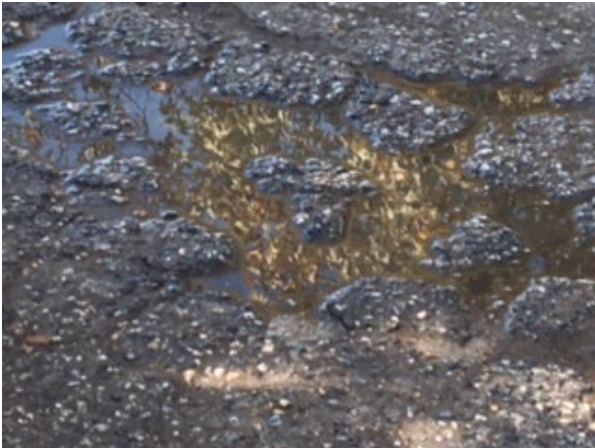
May need resurfacing, area near or in front of Café
