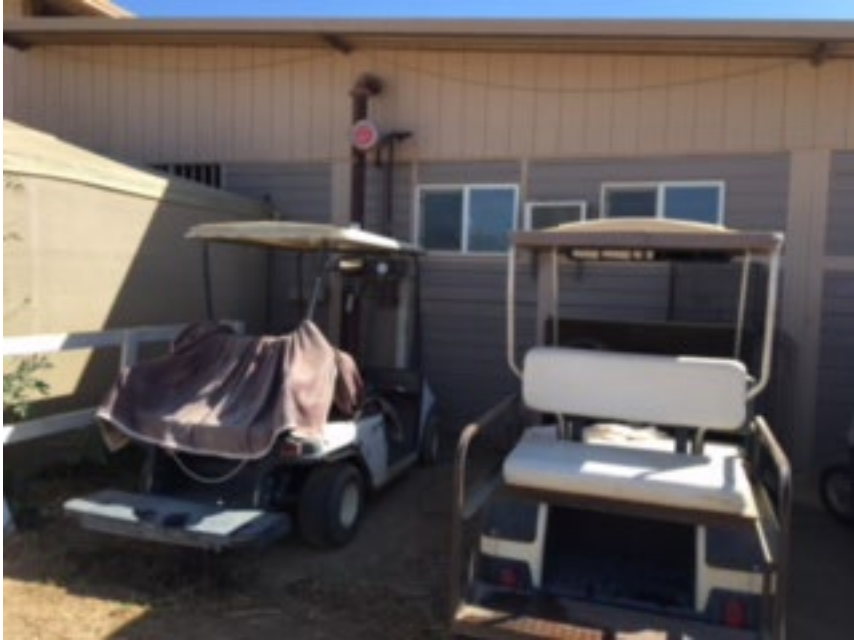
Golf carts blocking access to flow valves. Recommend moving cart.
