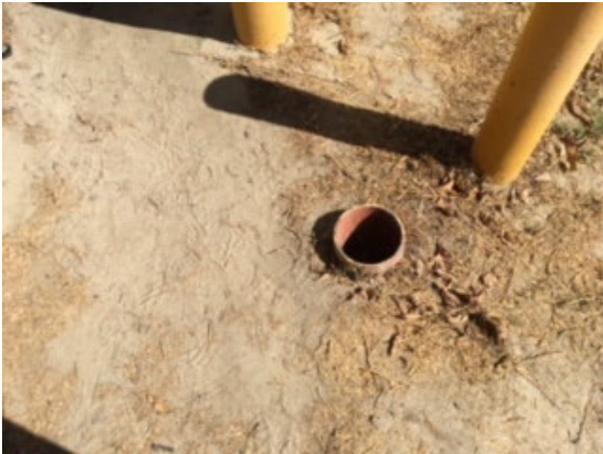
Hole need to be filled or removed, near East entrance gate above.
